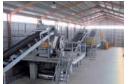
»8 Roller mill line with three roller mills installed in series
