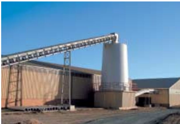
»10 Clay silo AGR 65c, supply belt with weather protection cover and lateral gangway
