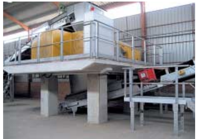
»9 Beta roller mill, WF 10120e, supply belt conveyor with Synchro material distributor, discharge belt with metal detector
