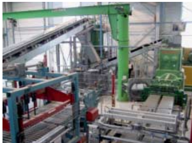
»13 Shaping plant: combined de-airing extrusion unit with twin-column exit, with the swung out second pressure head seen on the left, in front the cutter and the repositioned second cutter
